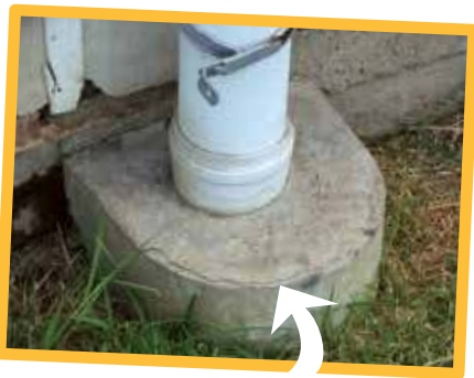
DT surround (disconnecter trap)
