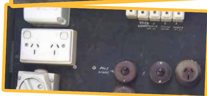
Zelemite backing board to an external switchboard
