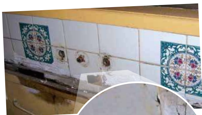
Ceramic tiles on asbestos sheeting
